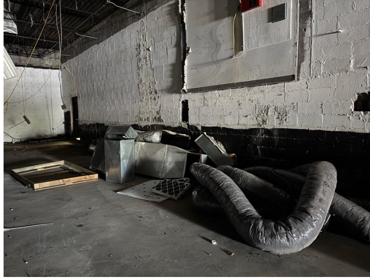
Above: Trash and debris remaining in building.
