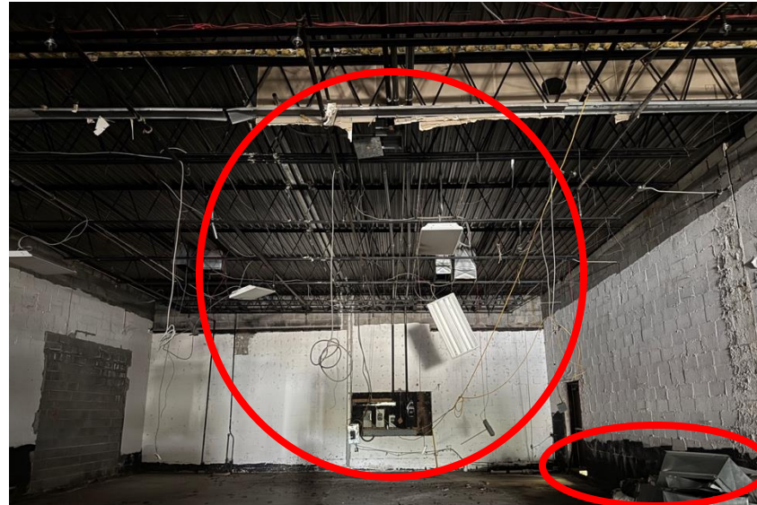
Above: Unconnected and hanging lights, exposed wires, and trash.
