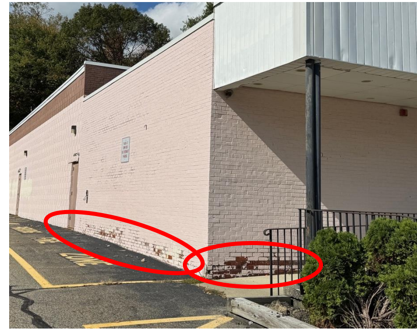
Above: Front and southern side of building with missing masonry and holes in the exterior wall.
