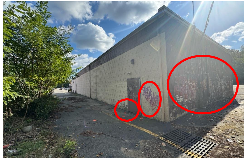
Above: Rear and northern side of building with extensive graffiti, missing masonry and deterioration of the exterior door.
