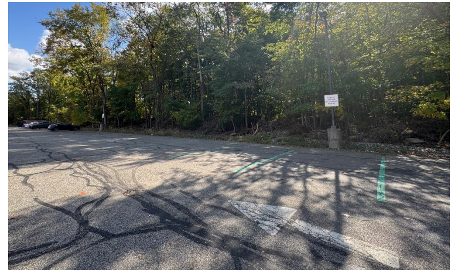
Above: Parking lot in poor condition with no stormwater detention/retention.
