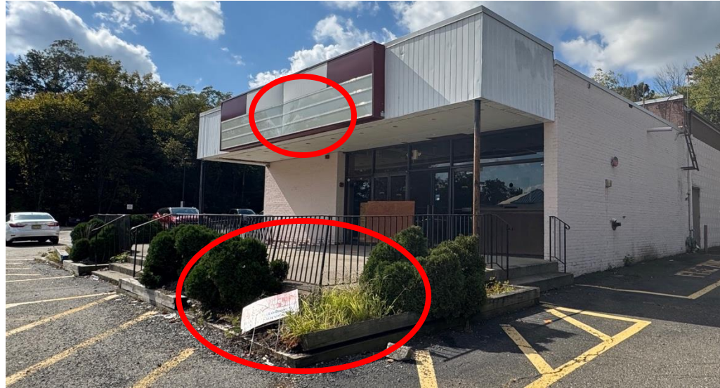
Left: Building front, facing south, with dents and a collapsed planter bed.
