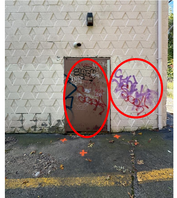
Above Graffiti on northern side exterior door
