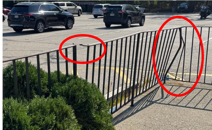
Above Front railing in need of replacement
