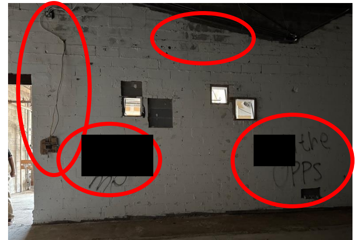
Above: Graffiti, exposed wires, dilapidated wall condition and graffiti (graphic graffiti has been redacted).
