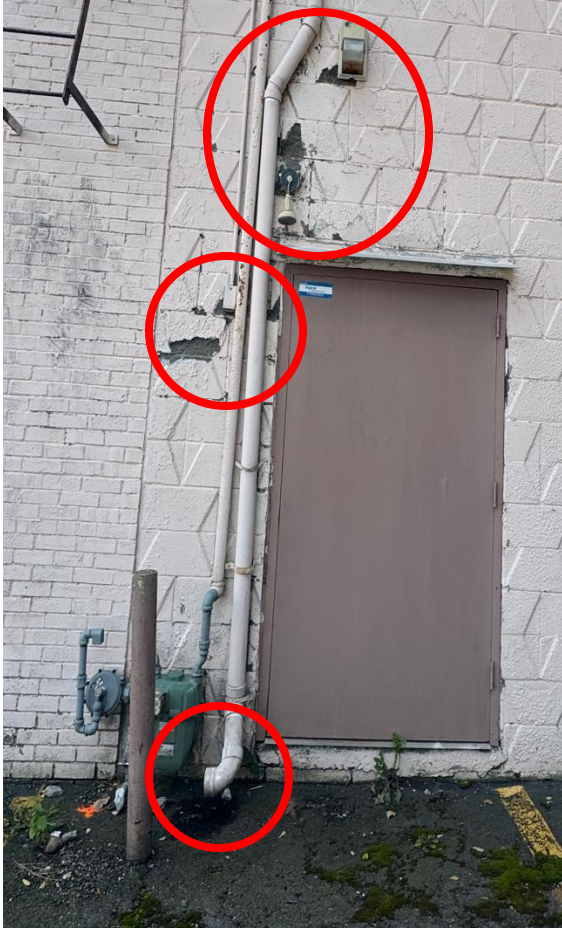
Left: Northern side of building with masonry loss and holes in the building exterior, as well as a gutter which empties to parking lot without collection.
