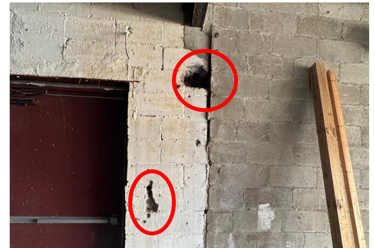
Above: Holes in the building interior wall.
